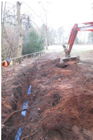
Water pipe comes through the site !!
